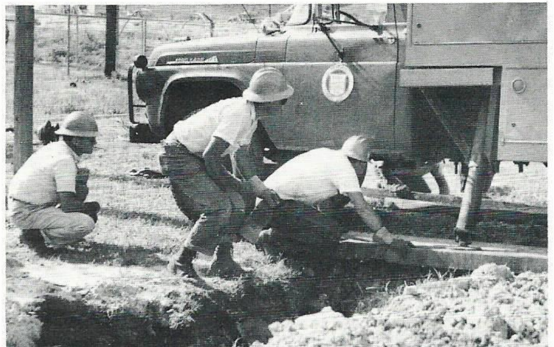
SETTING THE BRACES. Fabian Daigle, squatting left, watches as other Gulf Staters position timbers for the braces on this bucket truck in the yard at the Crown Zellerbach plant. The truck straddles an open ditch.
