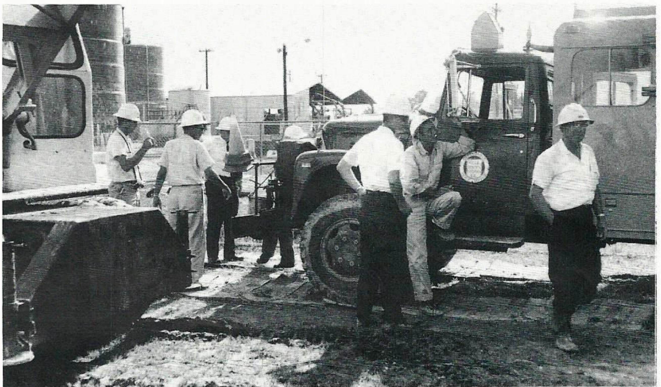
READY TO BEGIN LINE CONVERSION. This group of Baton Rouge Division line foremen and supervisors hold a last minute conference before the crews begin doubling the capacity of our electric lines to the Crown Zellerbach plant. The job was completed some 11 minutes less than the 12 hour outage the Line Department had requested of the big paper company.
