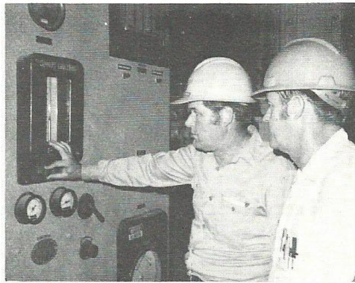
Johnson alters the gas flow into one of the boilers at the station.
