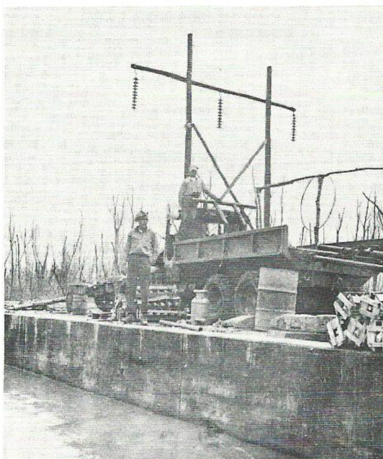
A floating workshop, this steel barge, with mounted winch truck, was used to hang insulators and string conductors.
