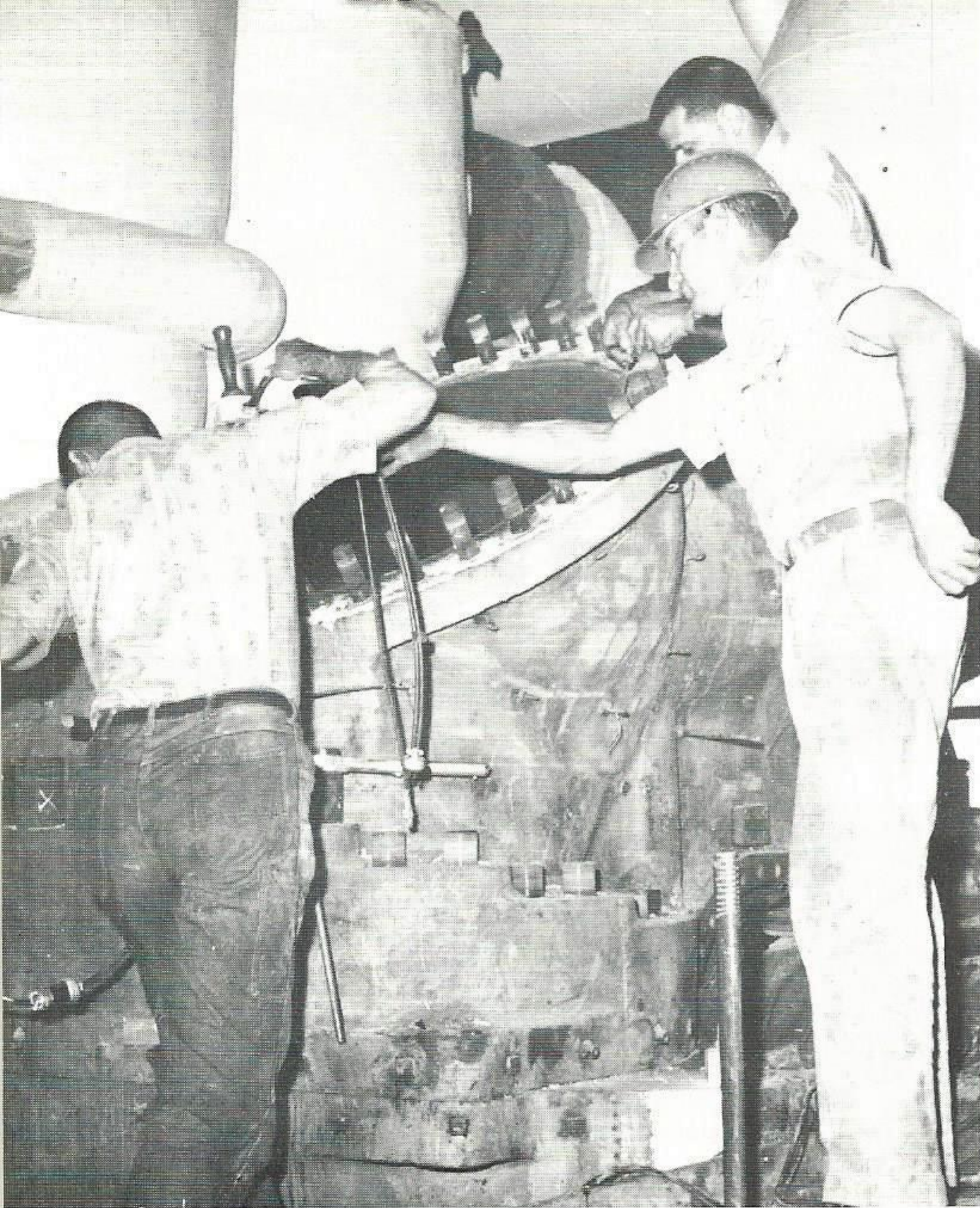
MOVING IN. With one of the crossover pipes out of the way, workers move closer to the center of attention: the turbine. Their next step is lifting the turbine cover. Shown from left to right are Steve Glach, repairman, first class, Neches Station; Frank Danna, electrician, first class, Neches Station; and Sheldon Fruge, repairman, first class, Neches Station. In the right background is Bill Martin, electrician, first class, Neches Station.
