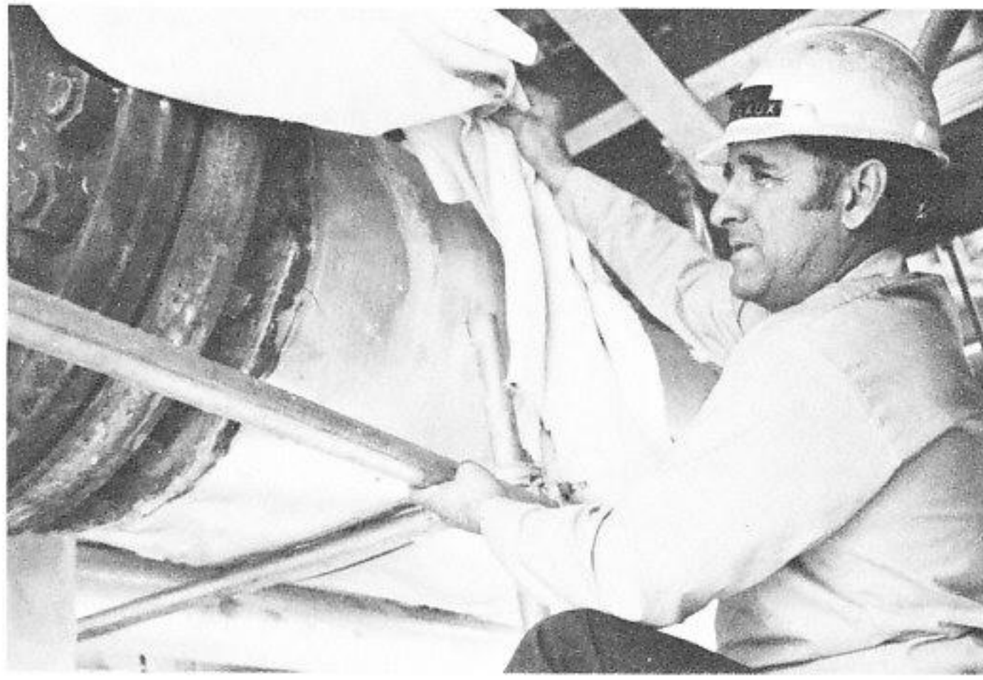
Scuddy Thibodeaux shows leaking connection.
