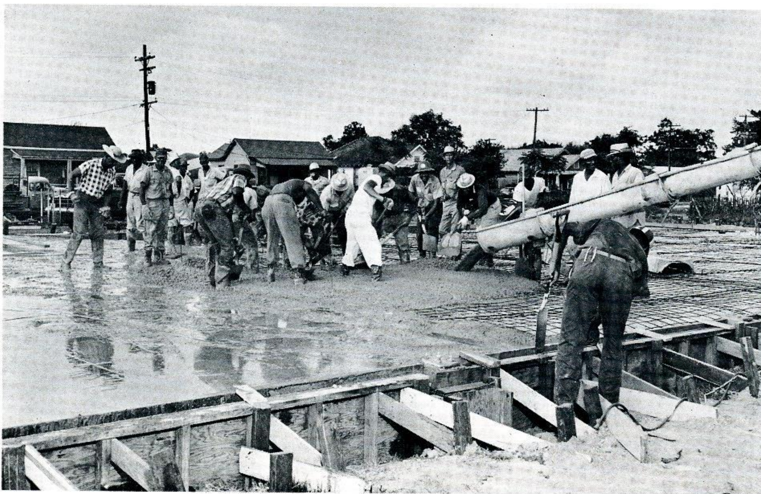
BUILDING GETS UNDERWAY. Members of the Beaumont Council of Knights of St. Peter Claver are putting in all their spare time to erect a new all brick building on the order's property. Here, on a recent Saturday, this group pours the concrete floor of the new building.
