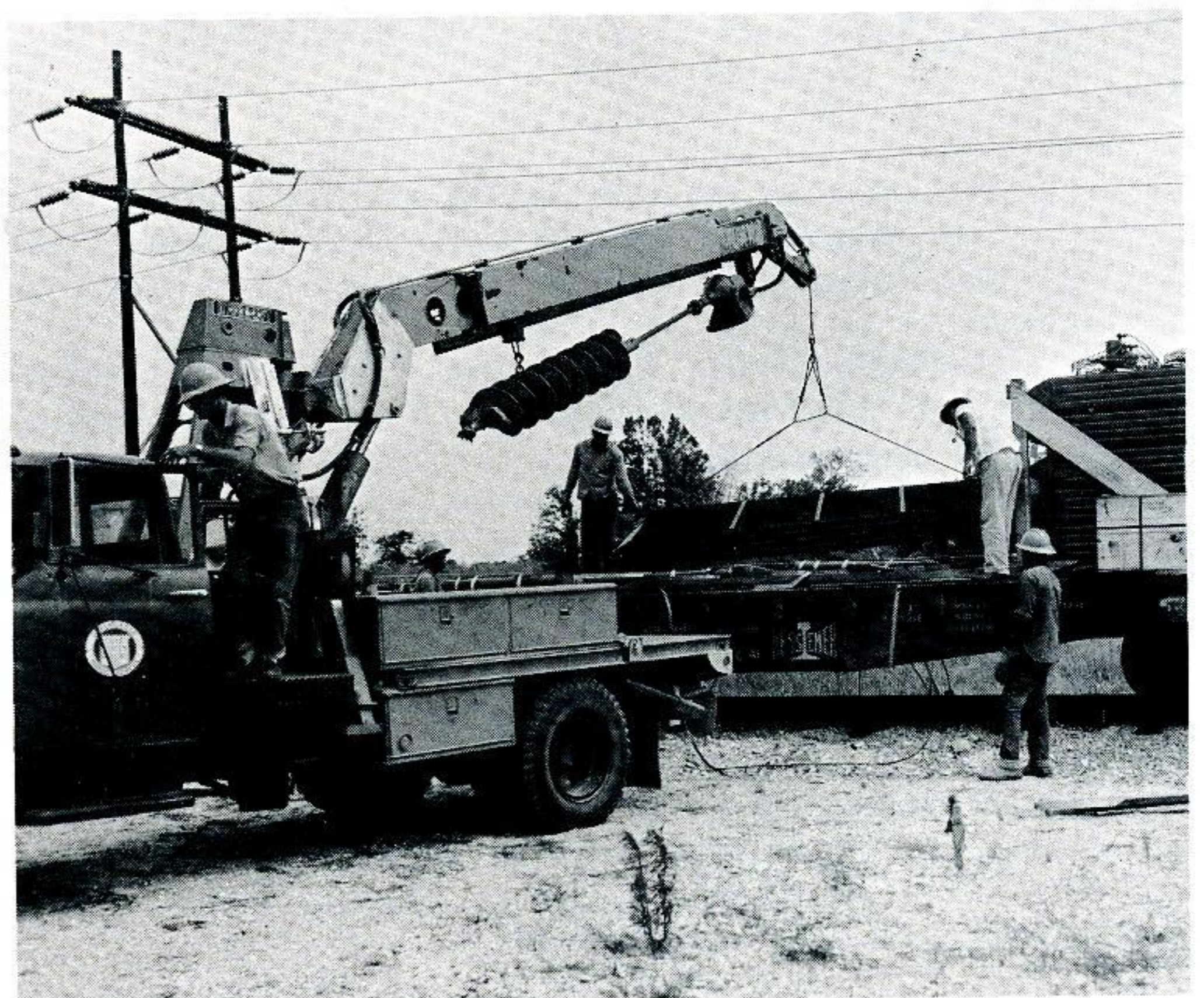
Attachments for transformer being unloaded from second rail car.
