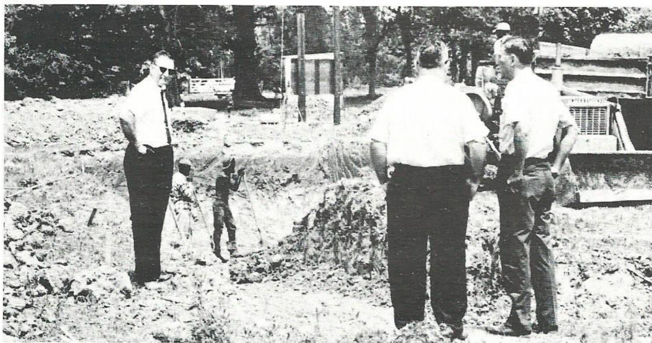
SWIMMING POOL UNDERWAY. Checking progress on the Baton Rouge Short Circuit Club's swimming pool are J. L. Clements and Jack Waltrip, Sales, and F. J. Gonzales, service foreman. The club expects to have the pool in operation by June 15. The members have been putting in the weekends clearing the club's new ten acre site and getting it in shape for use this summer.
