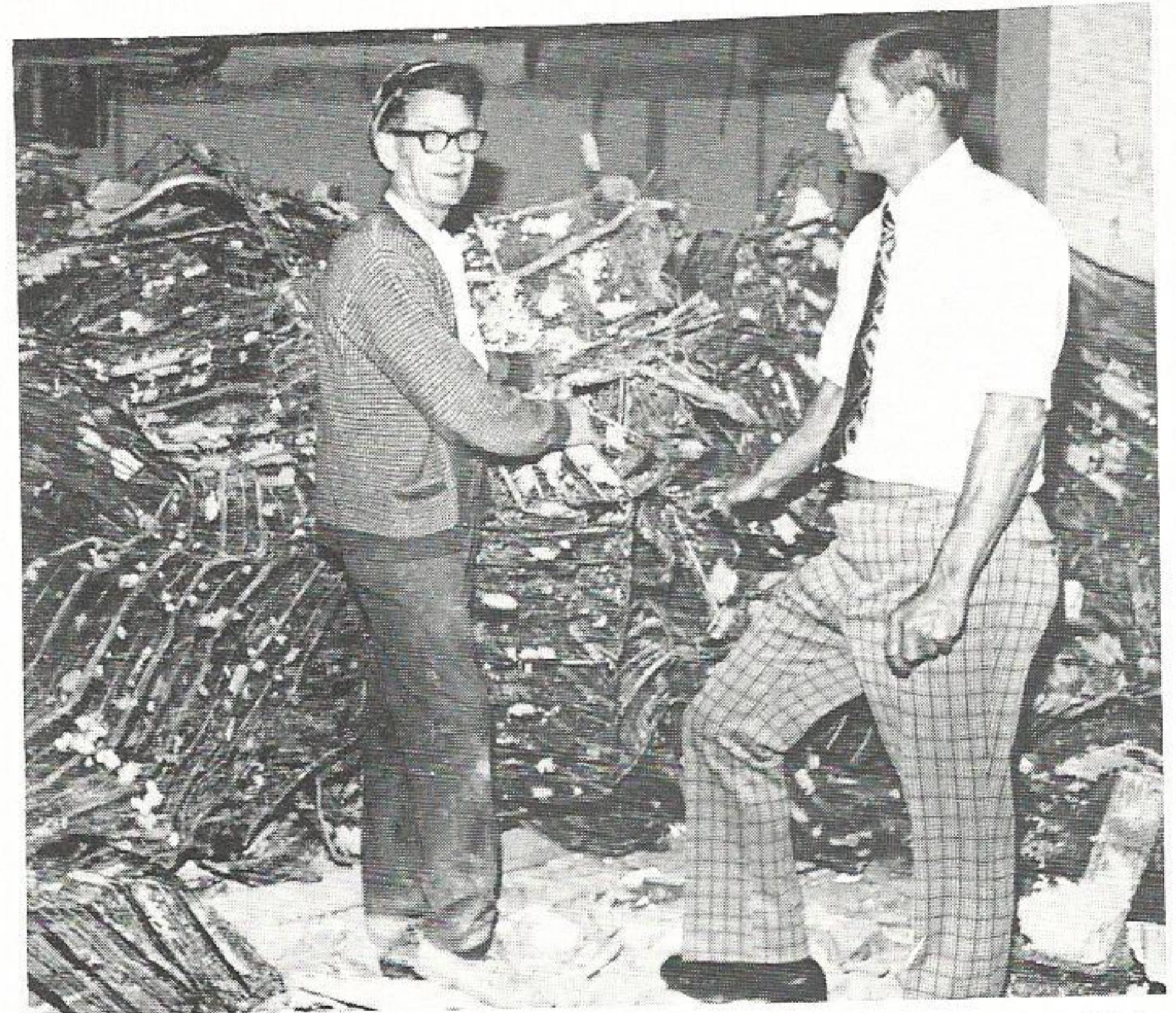
FOURTH FLOOR RUBBLE — The fourth floor of the Main Office has been "demolished" to allow remodeling into permanent offices of the system engineering, treasury and insurance departments. The area has been used as a storage room, janitors' meeting room and a junk room and had never been arranged for offices, according to Carroll Henry, building design section head. Above, Henry and Robert Odell Barclay, subcontractor for the job, pose near a pile of old plaster ceiling lath. The old ceilings and walls were broken into pieces and tossed down an outside chute (left) to a trash pile. Mike McCollum, whose wife, Cindy, is a clerk in plant accounting, handled the street-side arrangements. Henry said the total cost of the demolition and remodeling is expected to be about $180,000.
