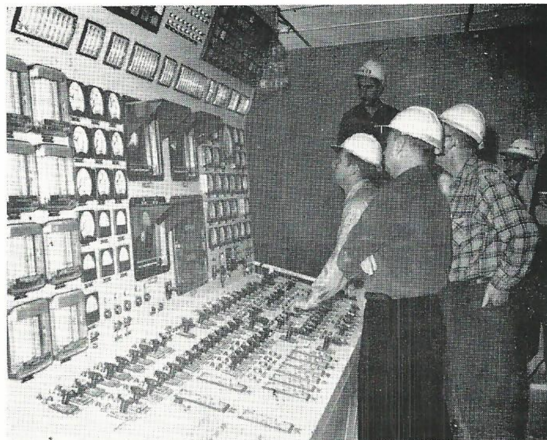
SWITCH ON. All eyes are turned toward Sabine Station's number one control panel as Walter Burris, center, control room foreman, throws the switch putting the unit on-the-line for the first time on January 31. Watching the board are: in background, Charles Gimon, office engineer; in the foreground, J. T. Graves, operations supervisor, Pat Sullivan, consulting engineer, Stone and Webster Engineers, and Bill Wilson, engineer, Production-Construction, Beaumont.
