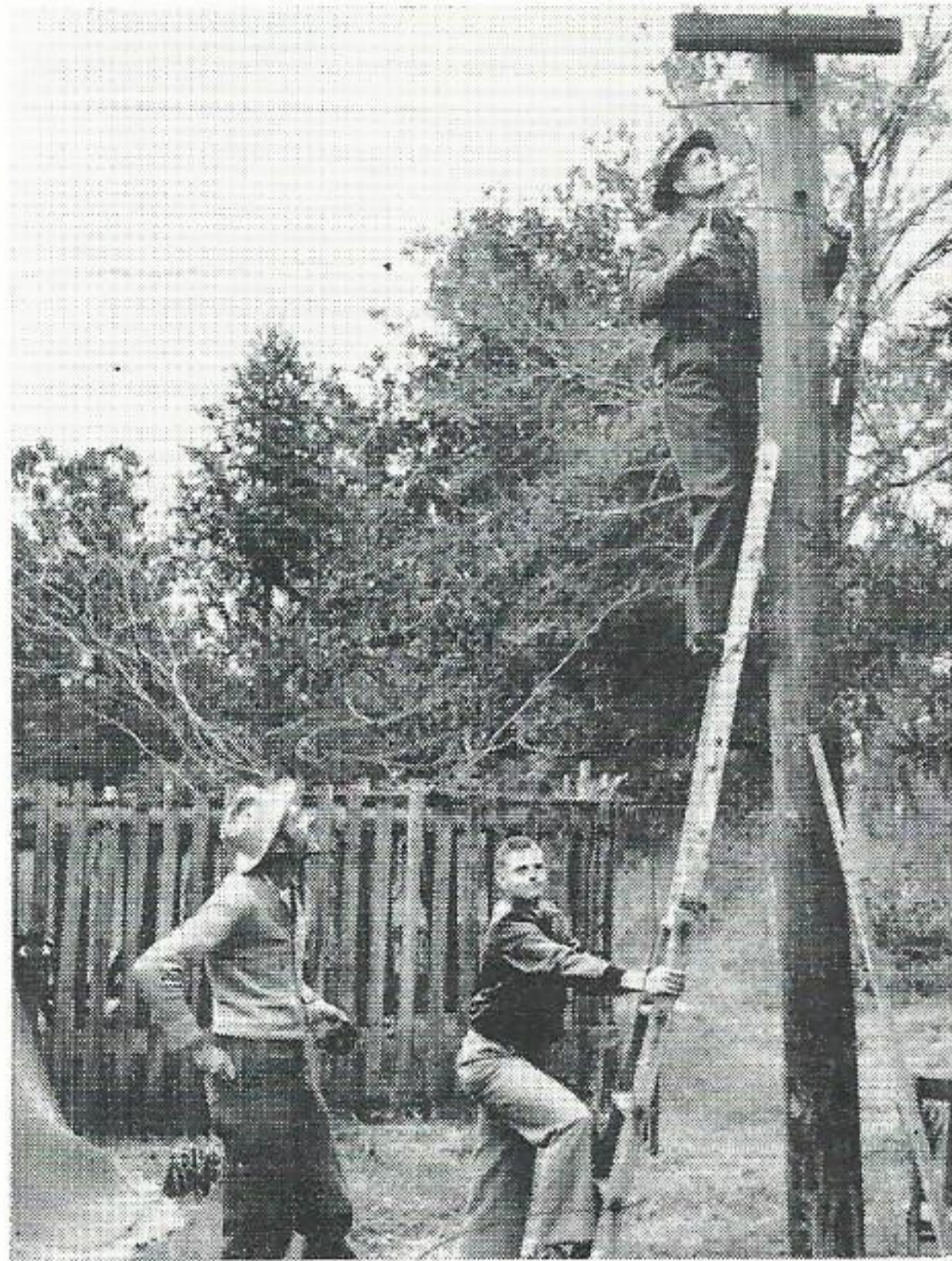
UP A POLE. Back in January, 1950, Aubrey Sprawls, bottom, and Vic Norvell, top, were on a ladder installing 220 volt service for a heating cable in a hot bed at the Watham Nursery at Shepherd, Texas. Watching them is Evan Watham, now a certified public accountant in Beaumont. Mr. Norvell is now district superintendent at Silsbee and Mr. Sprawls is area development engineer in Beaumont Division Sales.
