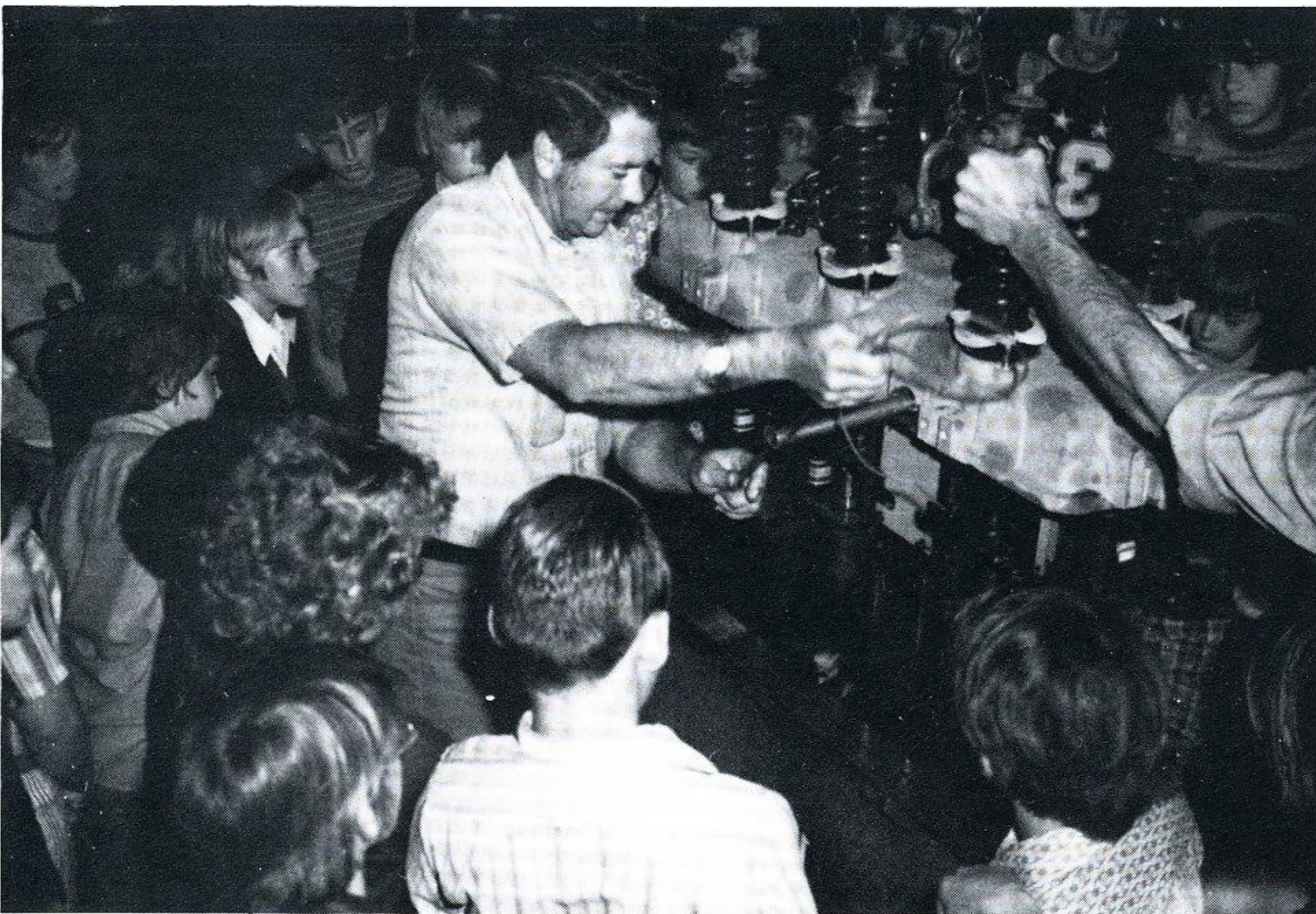
PRACTICAL TOUR — The fifth grade science class at Milton Elementary School in Lafayette was treated to a tour of Company facilities Feb. 26, including the pictured demonstration of the operation of a recloser by Edwin Judice, substation mechanic first class. The visit was coordinated by Toto Lacombe, residential sales representative. (from Bobbie Denais)
