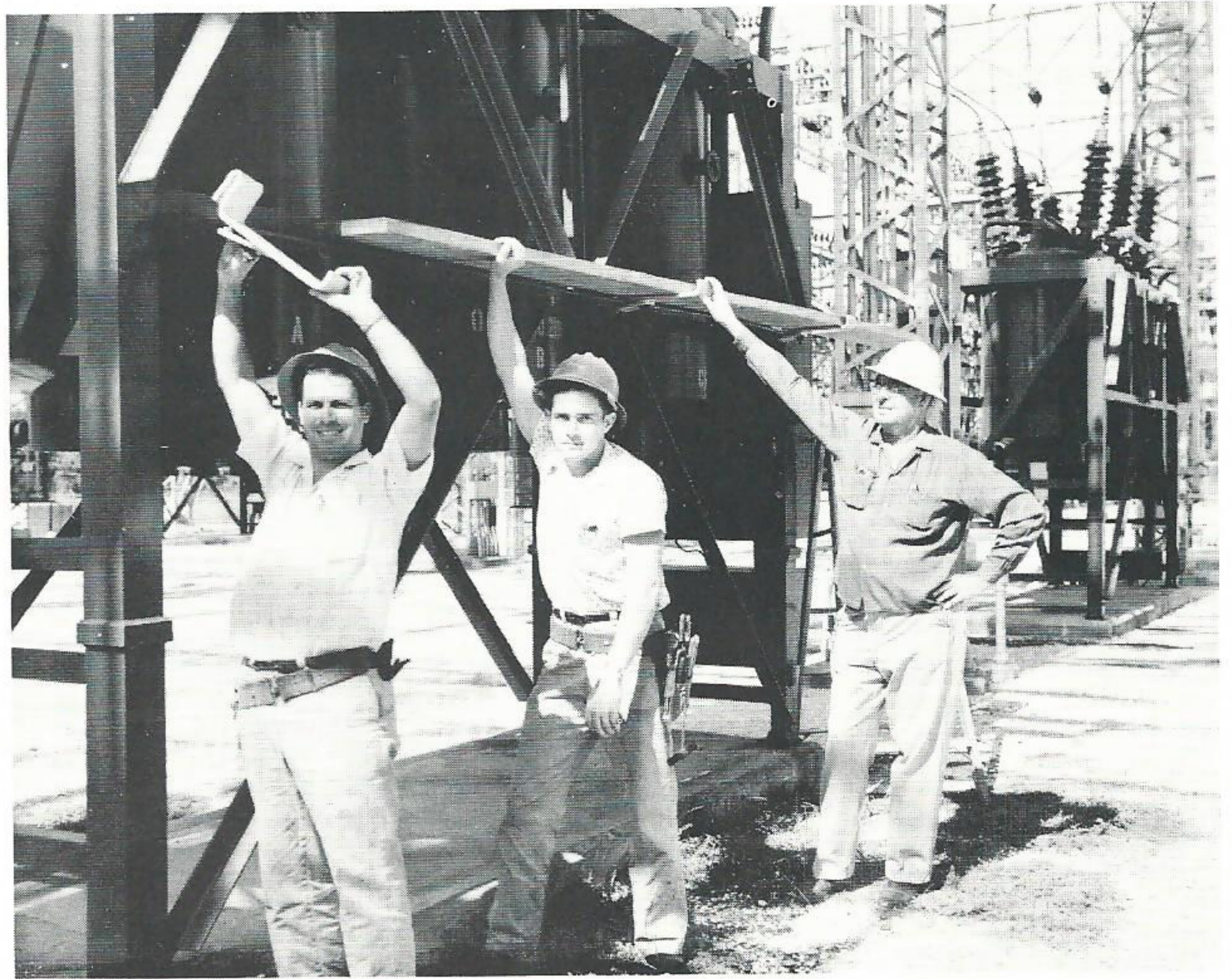
PUTTING UP PLATFORM. Bill Martin attaches third clamp while Bill Hale prepares to slide plank across to complete the newly devised work platform on an oil circuit breaker in the Neches Station substation yard. Both are electricians at the station. Prepared to assist with the plank is L. C. Pace, at right, electrical maintenance foreman.
