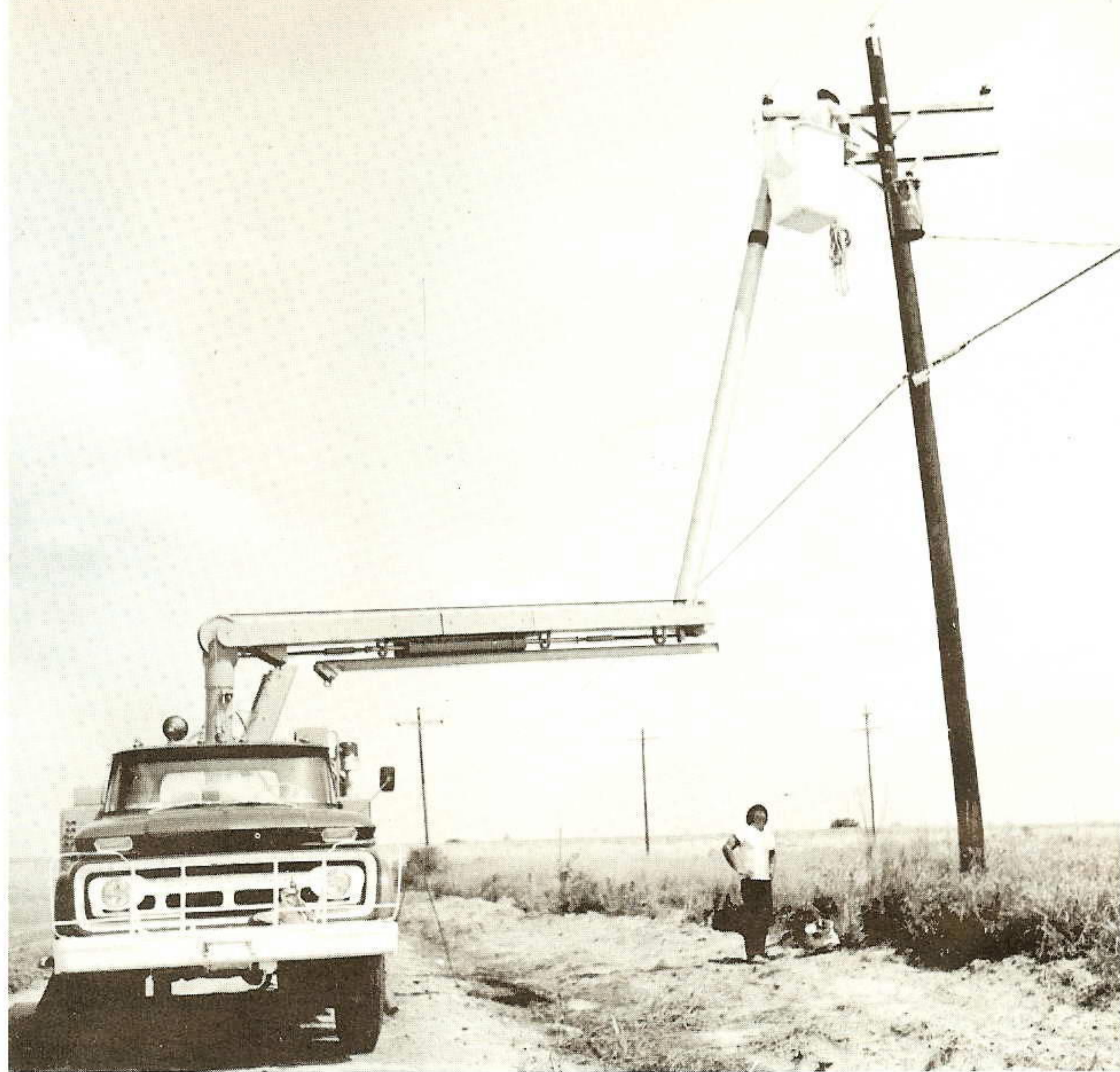
GSU'ERS AT WORK. O. J. LeBlanc, in bucket, and J. D. Breaux, both of Jennings T&D, were caught by the Plain Talks camera while servicing one of our rural facilities in Louisiana. Our Company's crews make numerous checks and service calls daily to insure dependable electric power to rural customers.
