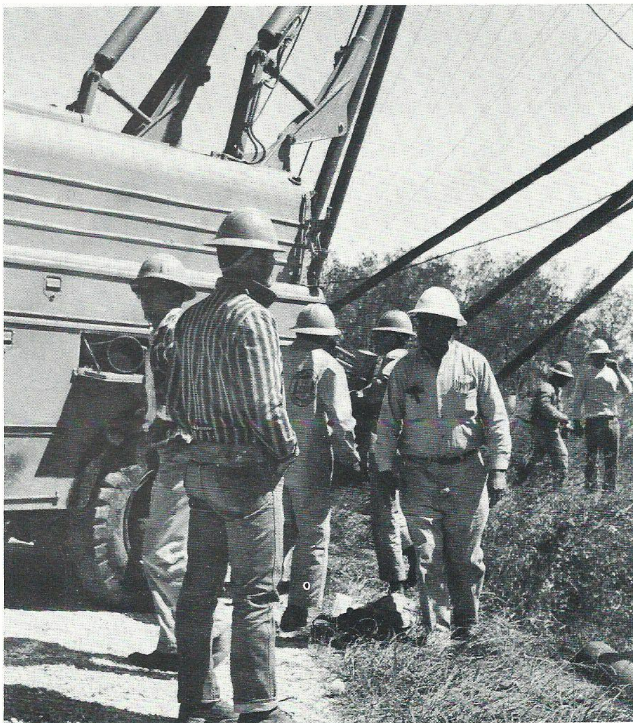
... the Port Arthur crew of Jim Minner helps restore service in Lafayette.
