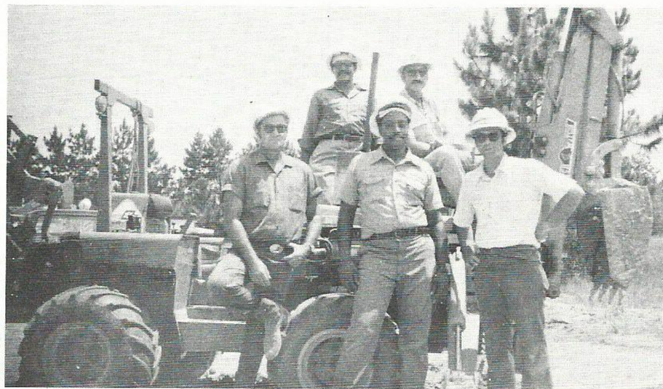
PHOTO BREAK — Members of this Lake Charles Division crew decided to take a quick "photo break" while working on the installation of underground service to a new subdivision. On top, left to right, are A. Henry and J. Manuel. Standing, left to right, are L. Cox, N. Slaughter and C. Berry. The new subdivision is called Country Club Acres. (from Edith Patterson)
