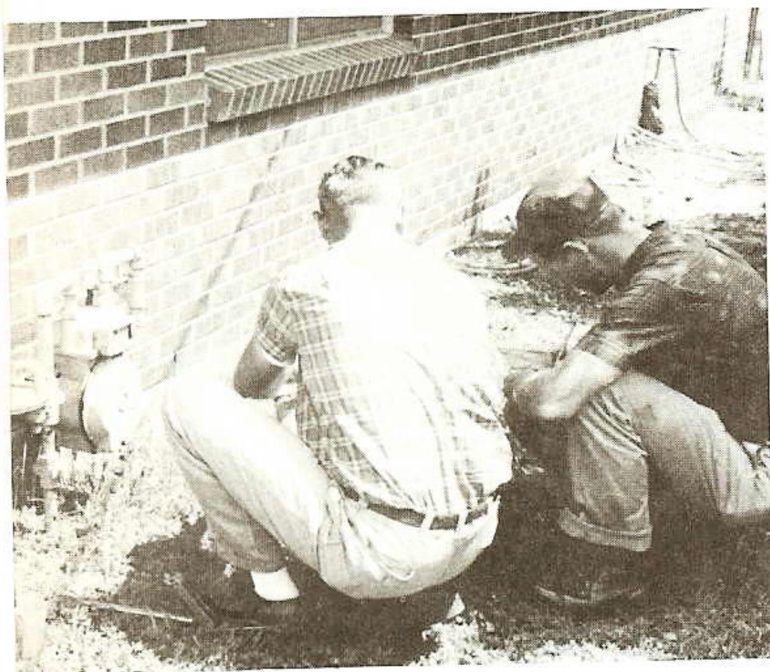
CHANGE OUT. Donald Kraft and Charles Siebert prepared a test tag on this residential meter before changing it out for testing in meter shop at the Gas Service Center.
